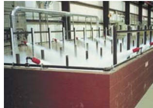
High Pressure CO2 Dip Tank Discharge.jpg
