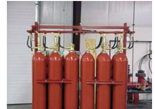
High Pressure CO2 Installation.jpg
