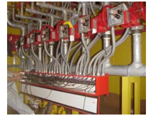
Low Pressure CO2 Installation.jpg
