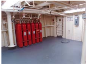
CO2 High Pressure Marine Installation 02.jpg
