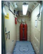
CO2 High Pressure Marine Installation 01.jpg
